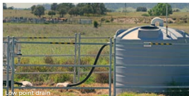
Low point drain
