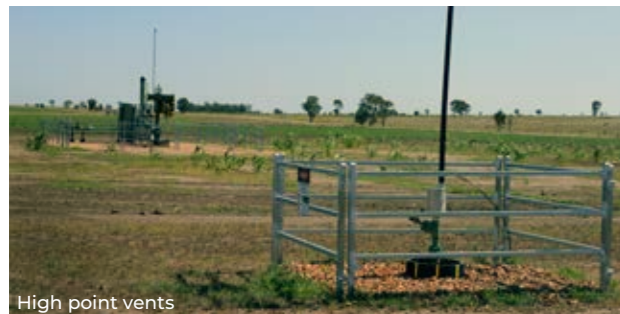
High point vents
